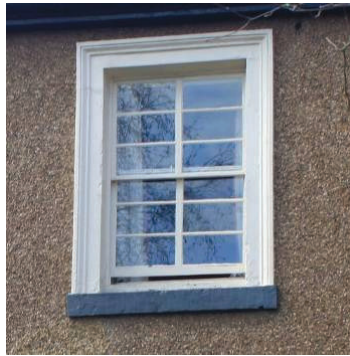
Double-hung sliding sash window with rectangular panes set horizontally and set back in moulded architrave
