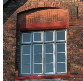
16 pane window having central inward-opening casements to lower portion and single-top hung casement to upper, with sandstone cill and lintel, set back beneath decorative brickwork panel beneath segmental brick arch
