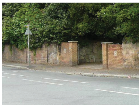
Inappropriate brick infilling and 'crazy paving' retaining wall behind
