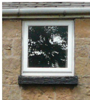
Early C19th plain small square window opening with sandstone cill set immediately under eaves, with modern window fitted
