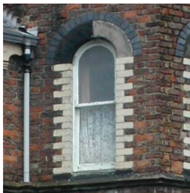
Two-pane sliding sash with segmental brick and sandstone arched head over projecting sandstone cill band with 'dogtooth' and polychromatic detailing
