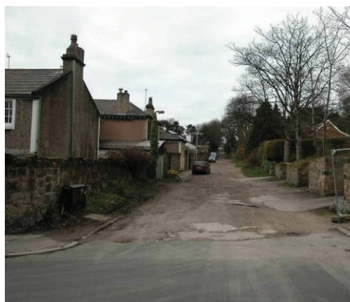
Arno Road West of Fairview Road is unmade, but heavy use has led to the creation of potholes and some uncoordinated patch repairs
