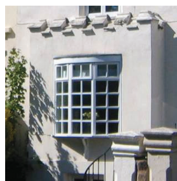
Modern bow window, probably replacing earlier 'flat' window set in crenellated bay structure.
