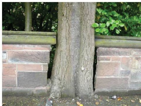
Low squared sandstone wall with copings demonstrating one method of retaining trees
